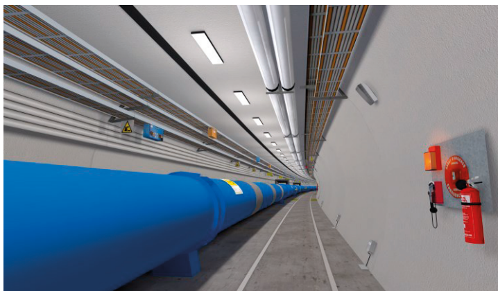
Figure 9 - View of the particle accelerator tunnel used in Experiment 4
