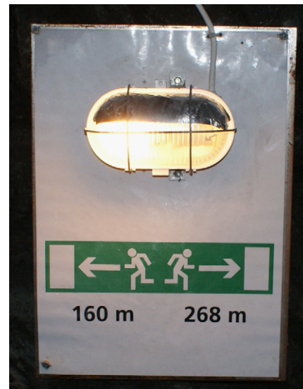
Fig. 2. A picture of the emergency sign installed every eight meters inside the tunnel.
